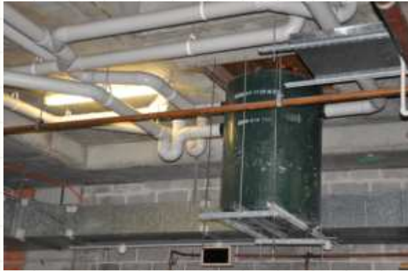
S100 suspended from a carpark roof
